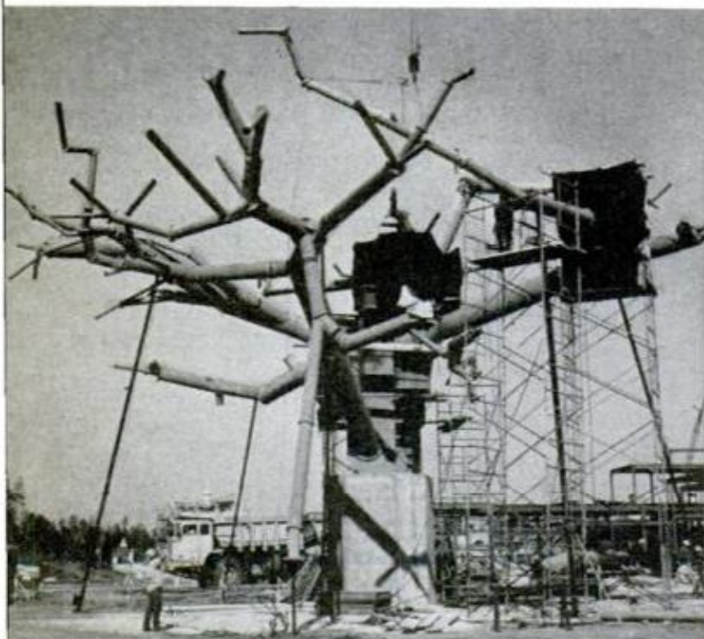
FANTASTIC TREEHOUSE "grows" in Adventureland with the help of a skilled crew of steelworkers
